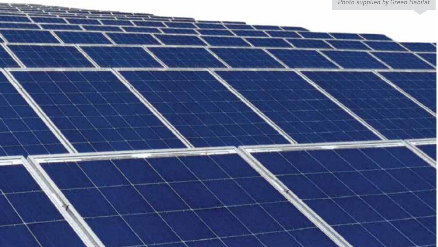
Photovoltaic installation on the Mustek building in Midrand Photo supplied by Green Habitat
